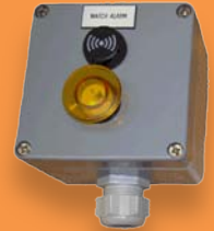
reset unit w. buzzer pre-alarm & alarm stage #1 engine room WAR 222.2.1.0
